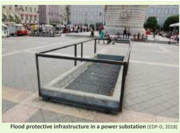
Flooding record inside power substation (EDP-D, 2018)
