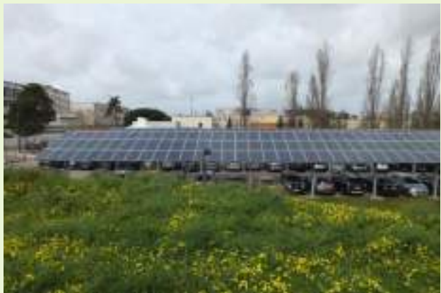
Photovoltaic panels in FCUL (CML, 2019)
